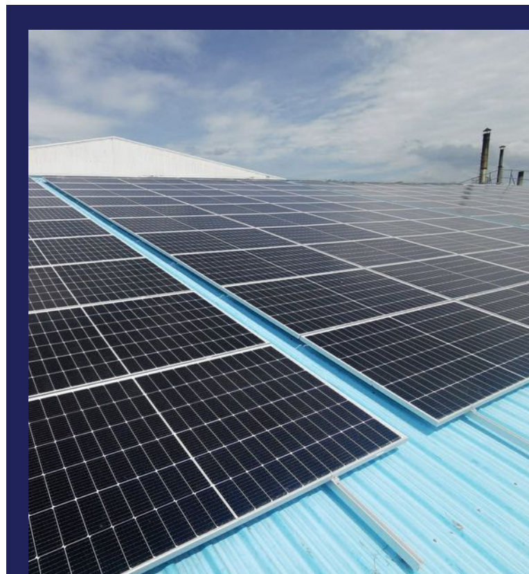
Solar panels at ASFII plant
